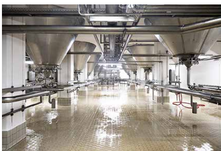
The beer ferments in the 39 huge storage tanks before it is pumped to the filling installation.
